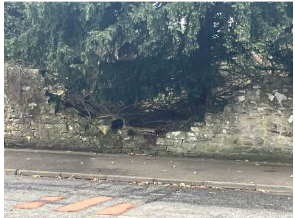
Figure 7.1: Collapsed section of Calder Estate wall, Main Street
