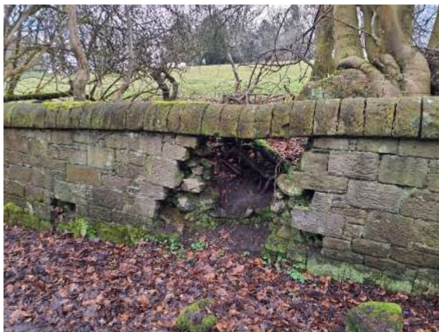
Figure 7.2: Example of damaged wall on Whitemoss Road
