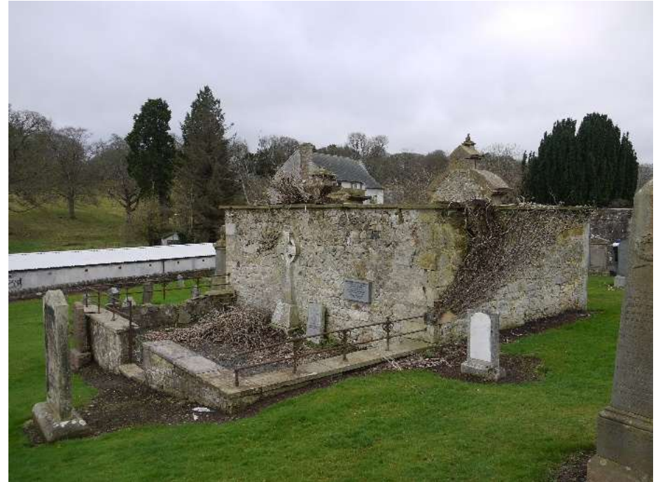
Figure 7.1: Dr. Cullen Burial Enclosure is in poor condition and requires repair
